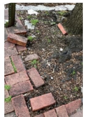
Loose bricks are an unsightly tripping hazard.
